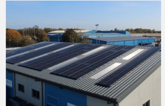
Figure 62: Image of the solar installation on Portsmouth City Council industrial units.
