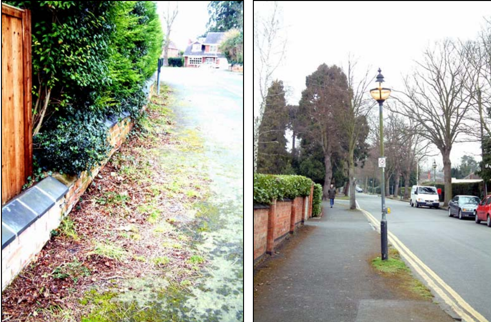
Plates 7 and 8: Poor pavement maintenance and Welcombe Road lamp standard
