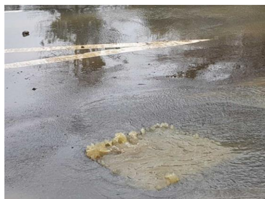
Images of flooding on the corner of Armscote Road and Front Street Including image of flood water coming up through a manhole cover
