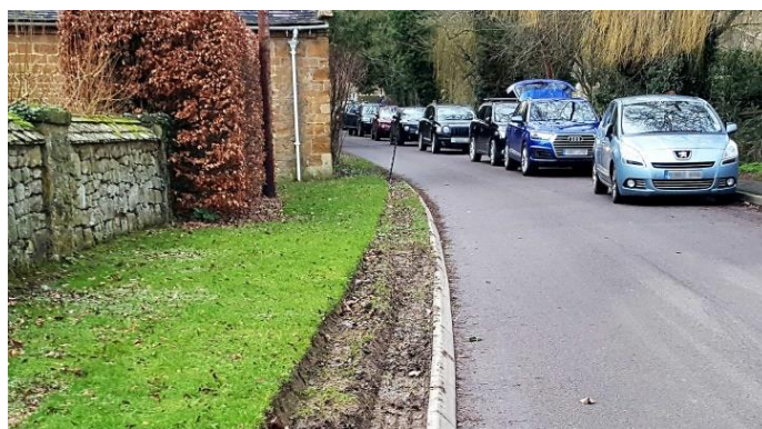
Verge damage on Back Street
