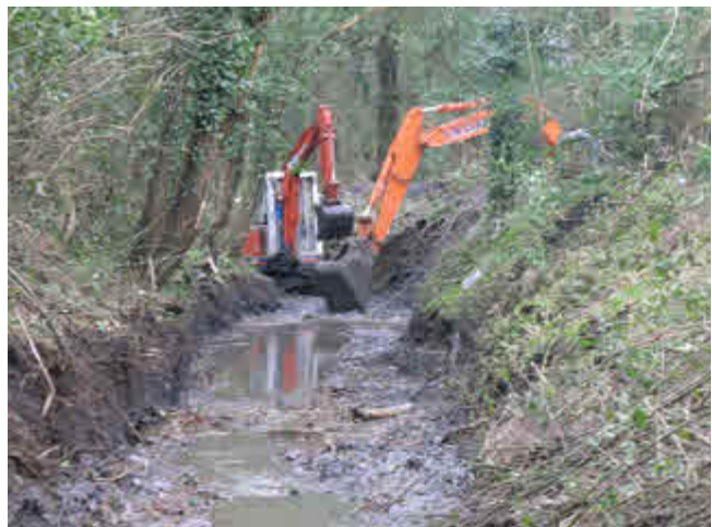
Clearing Lot Brook after the floods of 2007
