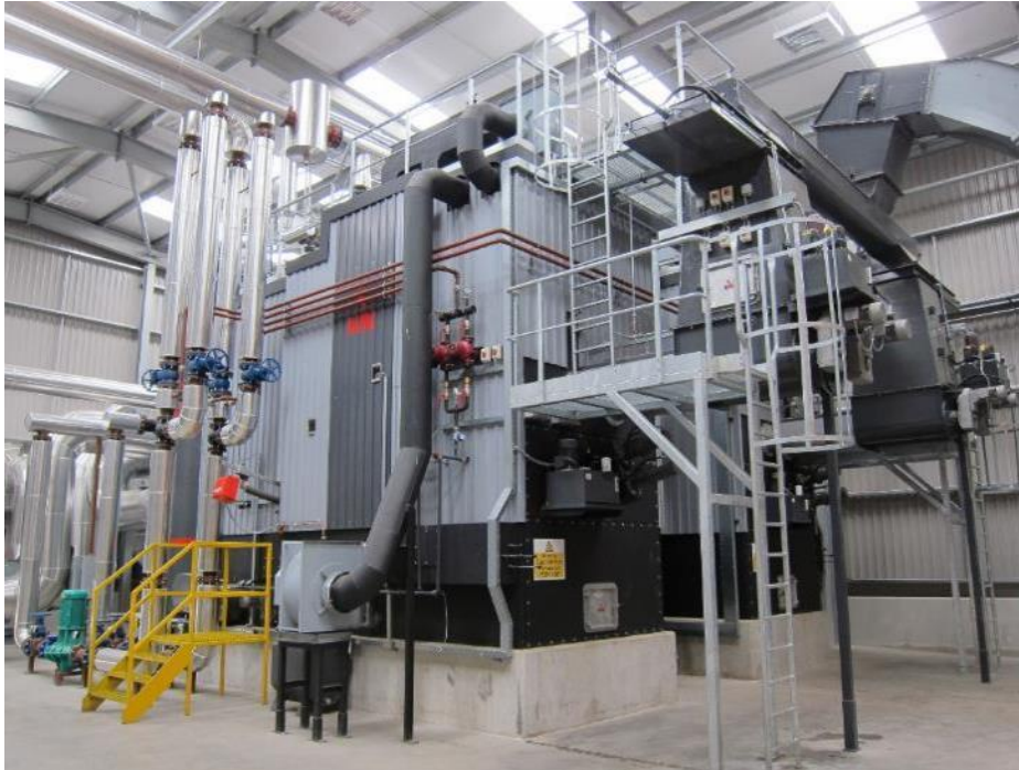
6MW Wood Chip Boiler at Sawmill Site in Mid-Wales, Photo Courtesy of Sustainable Energy Ltd
