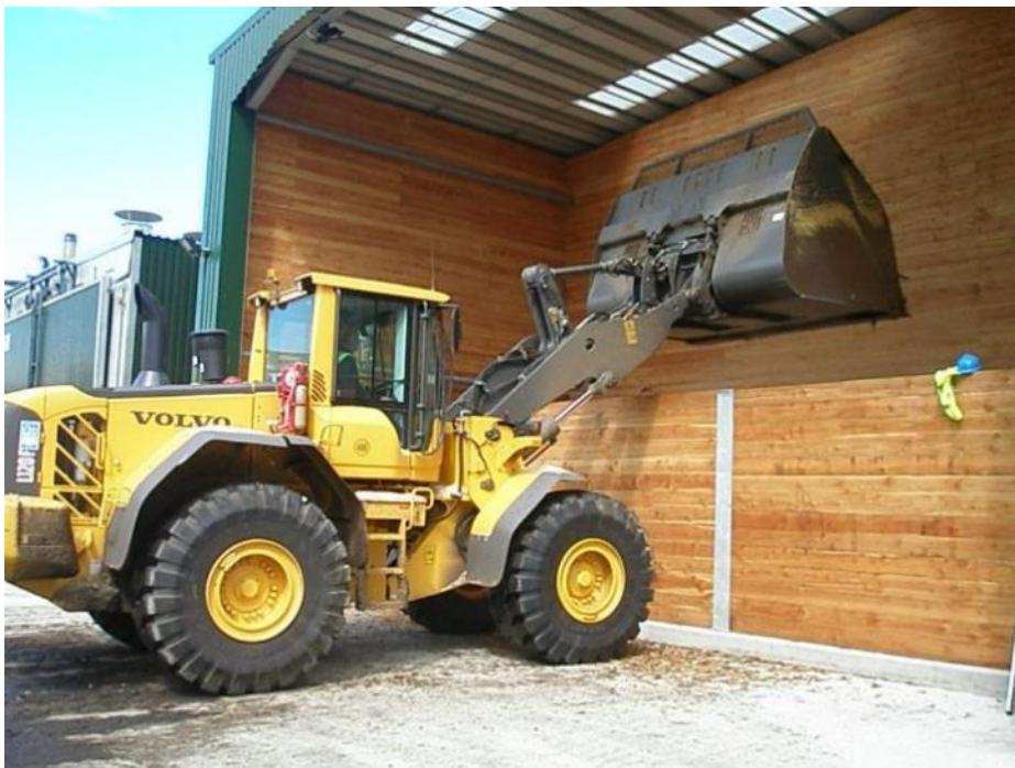
Wood Chip Delivery to Wood Chip Store for 6MW Biomass Boiler, Photo Courtesy of Sustainable Energy Ltd
