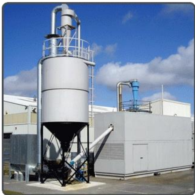
250kW Wood Gasification System, Photo Courtesy of Sustainable Energy Ltd
